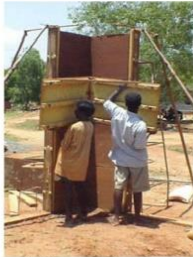
Lifting panels of the second form to the fourth one of a corner wall
