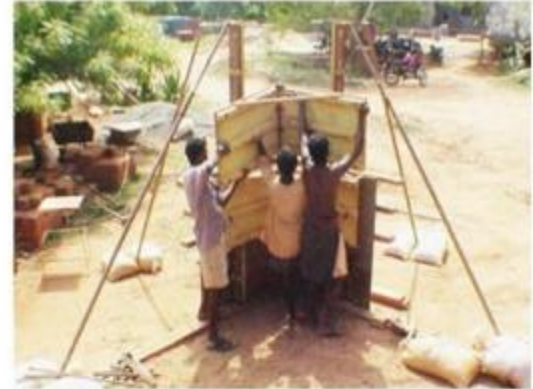
Lifting panels of the first form to the third one of a corner wall
