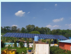
Solar power plant at Wai FSTP
