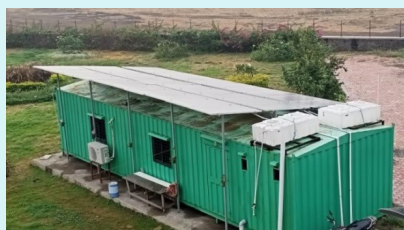
Solar power plant at Sinnar FSTP
