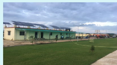
Solar power plant at Bhubaneshwar FSTP
