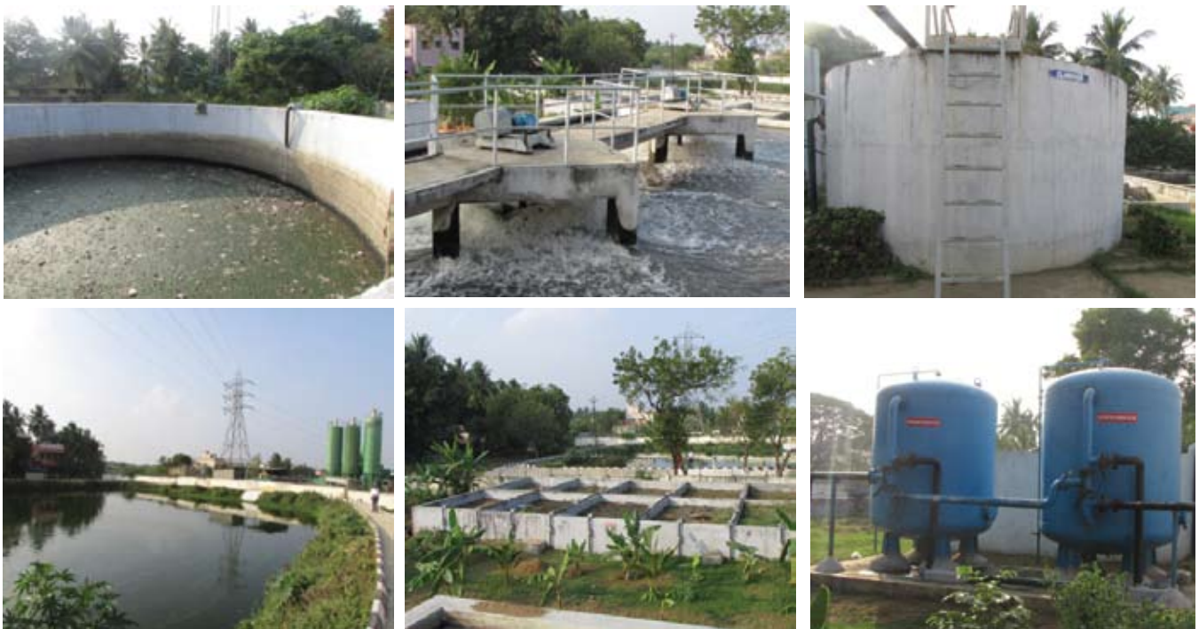
Image 2: (Clockwise from top left): Collection well; clarifier; settling tank; pressure sand and activated carbon filter; sludge drying bed, and treated water pond with walking track
