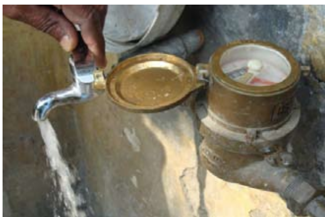
Image 1: Metered 24x7 water supply in a house in Paprala village, Ropar district
