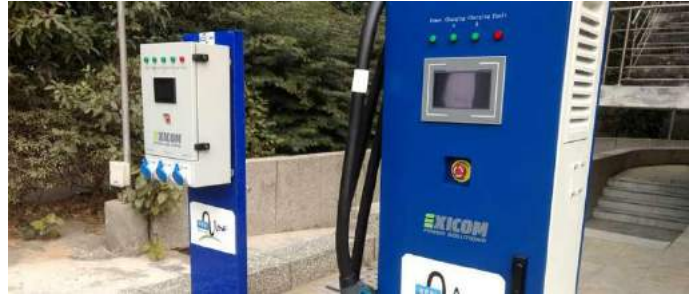
Figure 188 EESL Exicom's AC-DC charging stations for EVs
